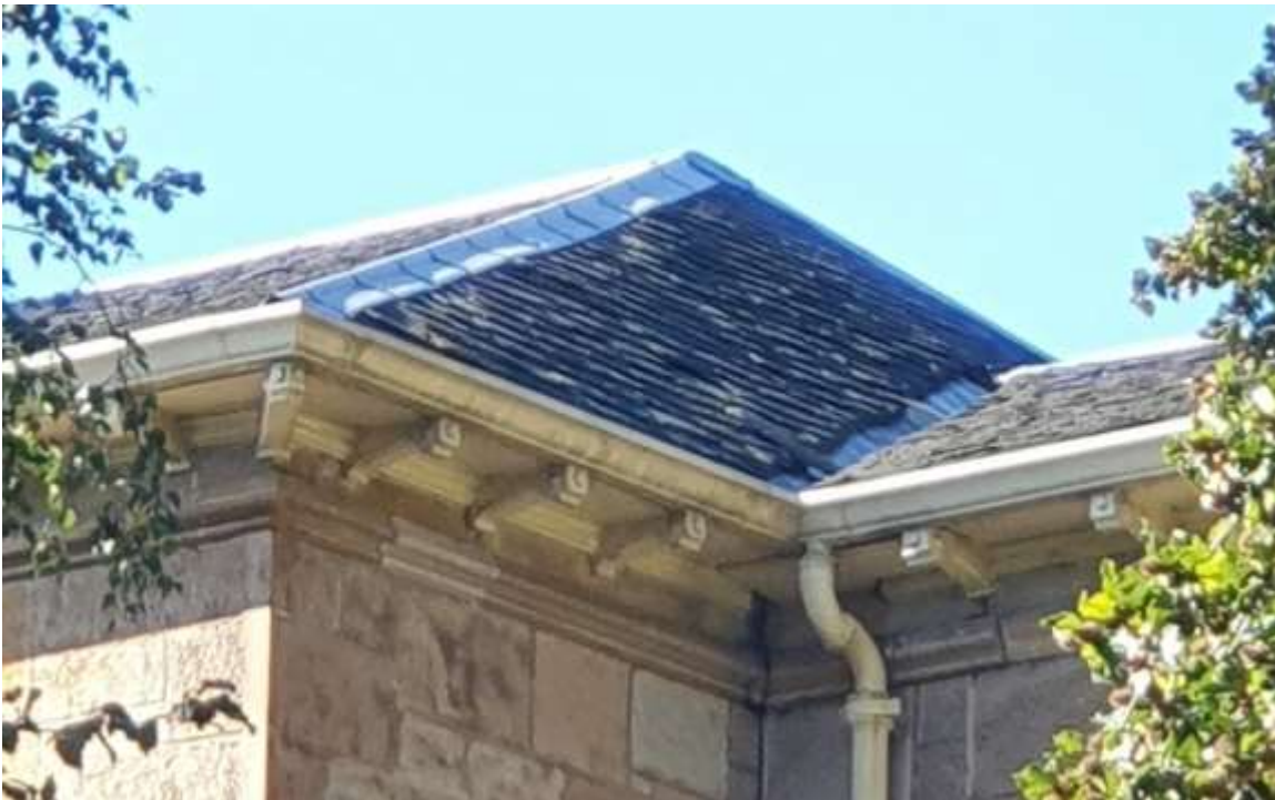
Plate 6. Roof at front of building (northern end), missing slates, gap under ridge etc.
