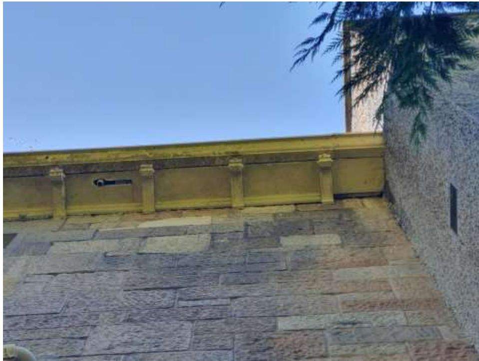
Plate 5. Northeastern gable of building – gaps in soffit and behind it
